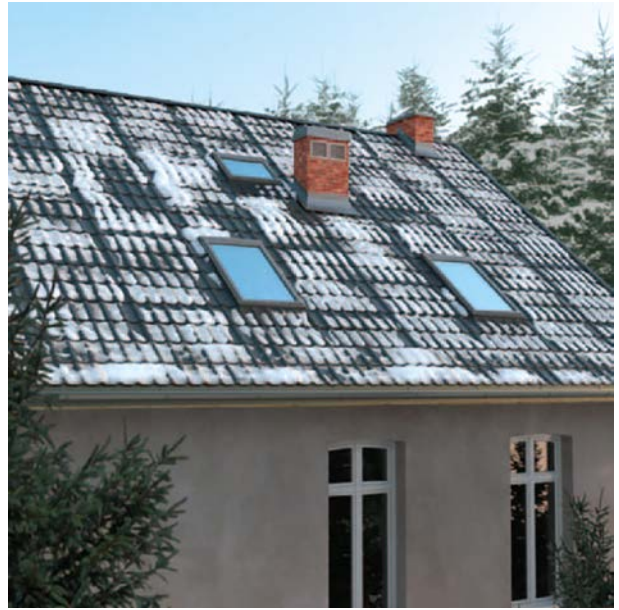
1.3. An example of thermal bridges - melted snow in places where heat gets through rafters on the roof
